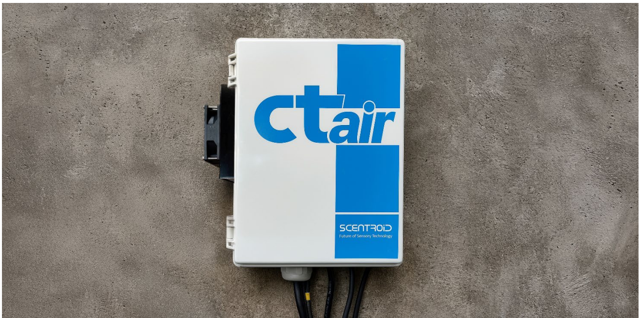
Wall-mounted CTair device equipped with an Air Conditioning unit
